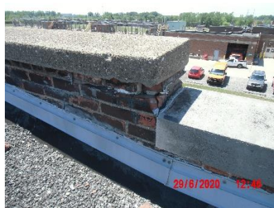
View of Coping Sealant (Black/Tan)
