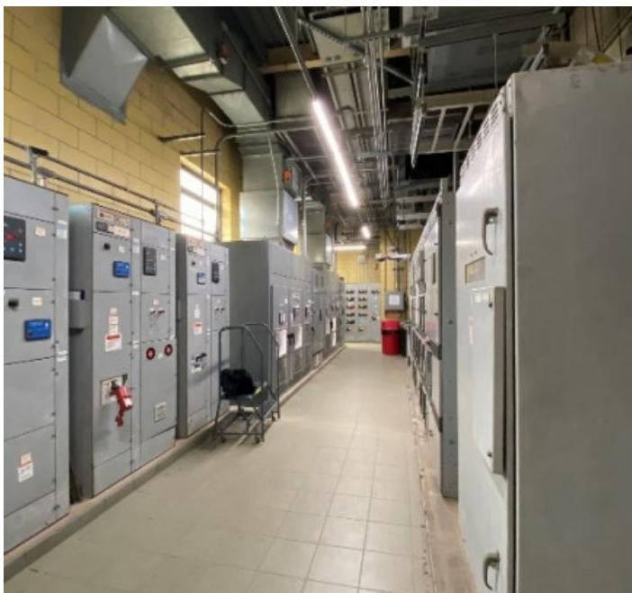
6C - IPS Electrical Room with Air Quality Concerns (None Found)
