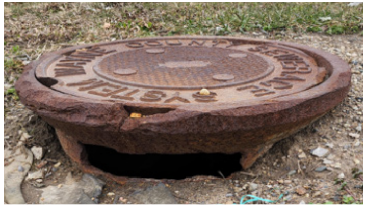
4C - Manhole Needing Repair
